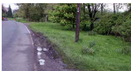
Verge damage in Mill Road
