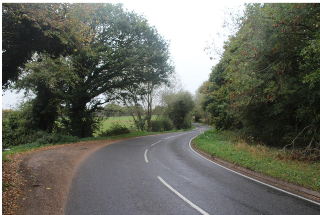
Figure 15 - Erosion and kerb stones on corner of Herbage Park Road
