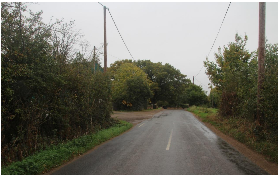
Figure 13 - Erosion and widening at farm entrance
