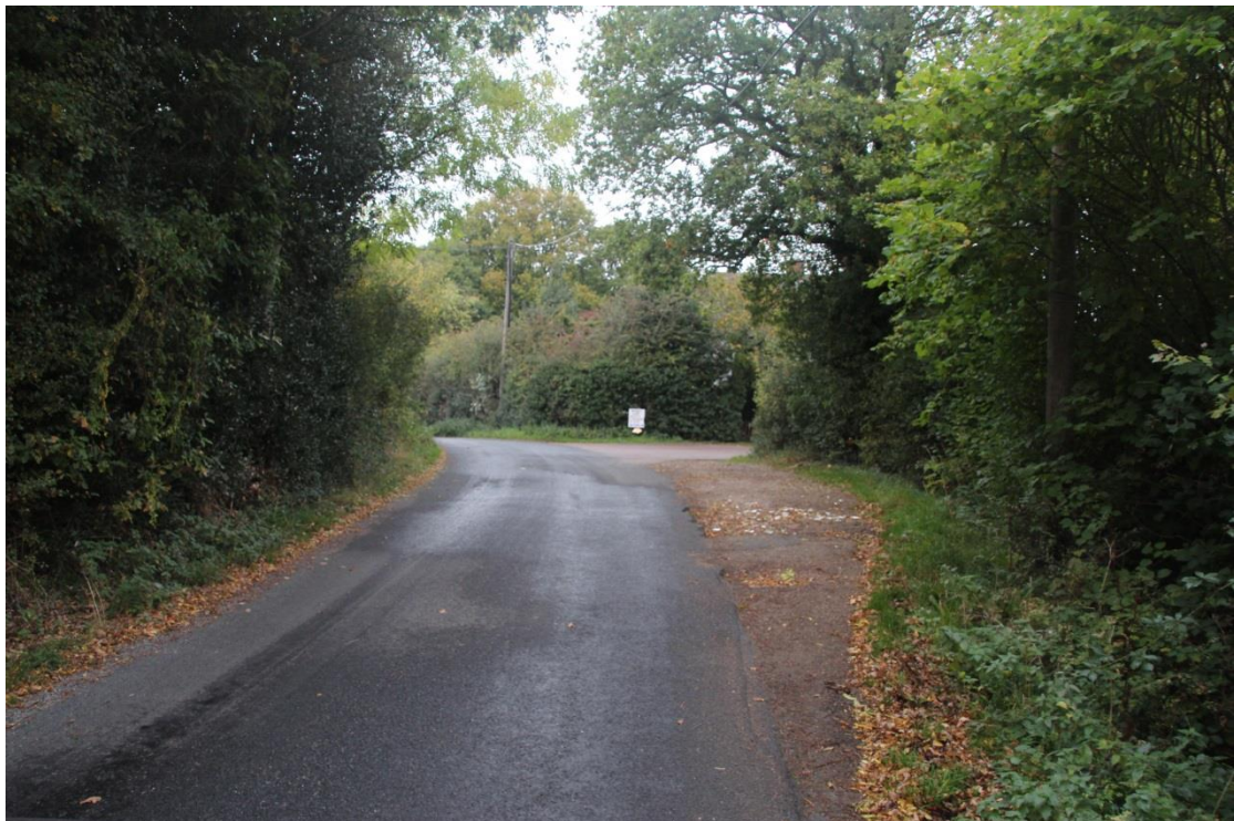
Figure 7 - Erosion in passing/parking space on bend
